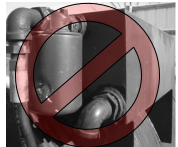
NO LEAKING HYDRAULIC HOSES!
